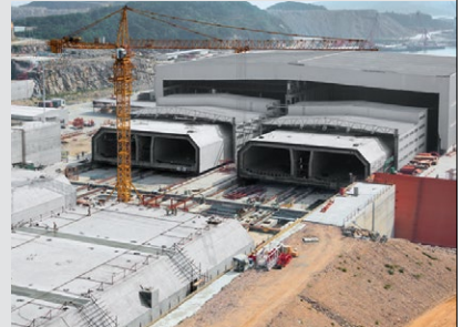
Tunnel tubes are moved from the field factory, sealed with bulkheads and installed on the sea-bed.
