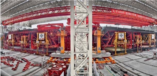
Two hydraulically-operated shuttering machines in use for the realization of 180 m long tunnel tubes with incremental launching.
